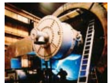
Figure 3.15 Both generators have coils that rotate in a magnetic field.
